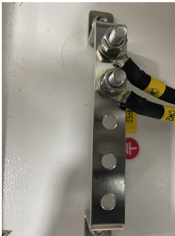
Figure 20 Ground copper bar
