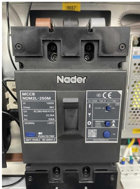
Figure 8 Main circuit breaker
