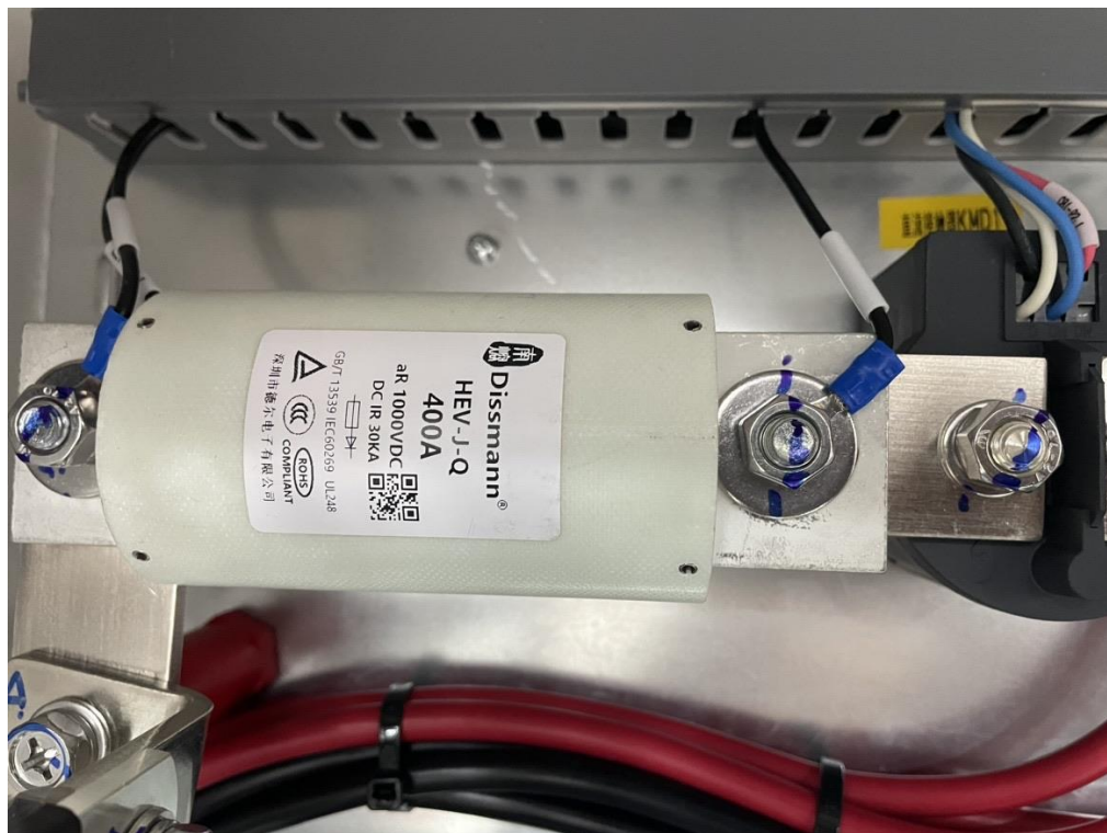
Figure 12 DC Fuse and DC Contactor
