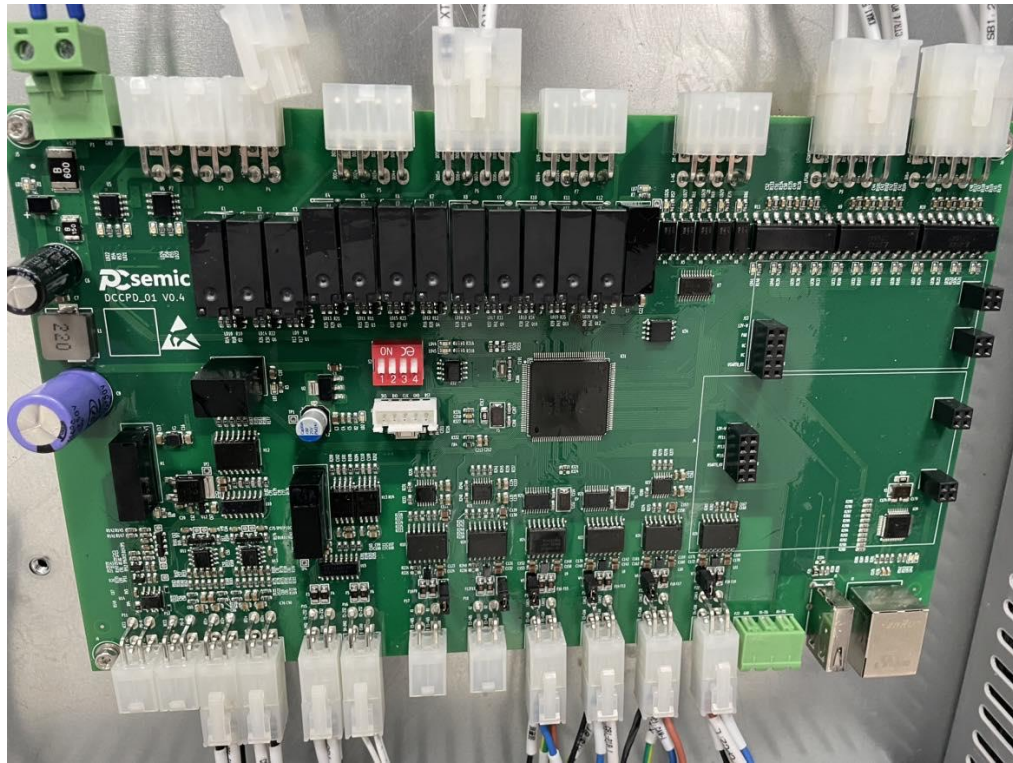
Figure 17 Main control board
